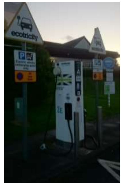
Electric Charging Points at Service
